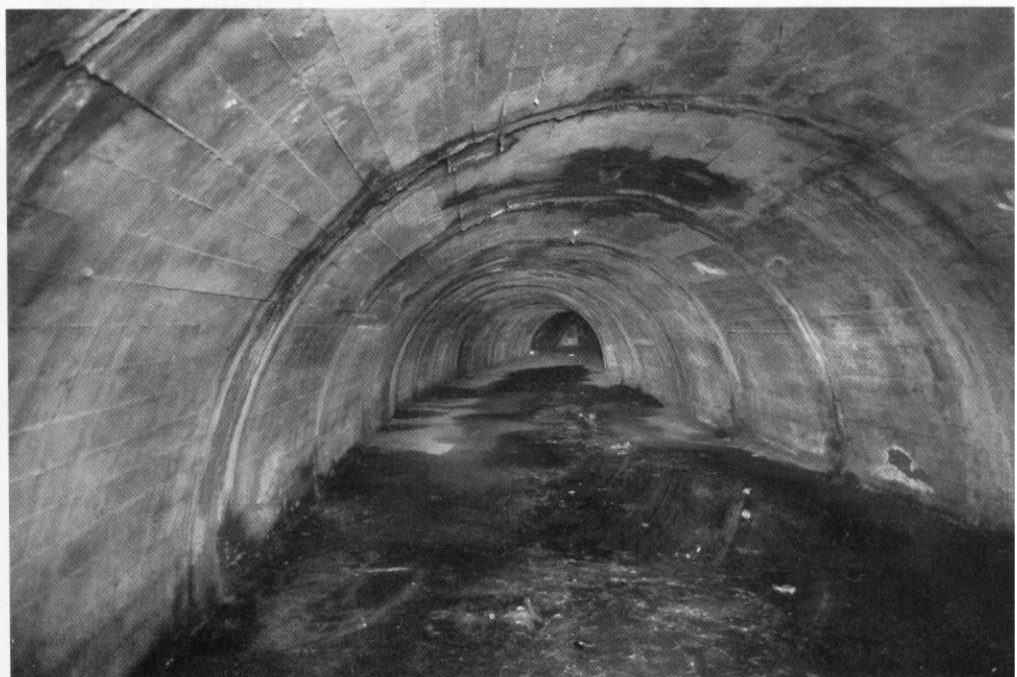
The specially raised floor of the 1940s air-raid shelter ends after 650m , and then the original lower culvert floor is exposed as seen here
